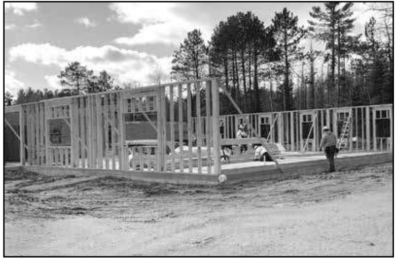
New Ranger Station rises from site of its historic predecessor. Photo Mike Hittle
