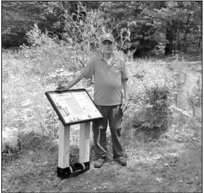
Boot Brush installation, ICORE volunteer, at Hidden River Trail, photo by WDNR Staff.
